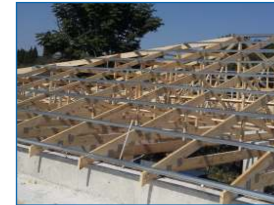
40mm Top-Hat profiles used as metal sheeting purlins on timber roof trusses.
