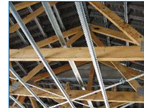
20mm Top-Hat ceiling branding installed on timber roof trusses with a concrete tile roof covering.
