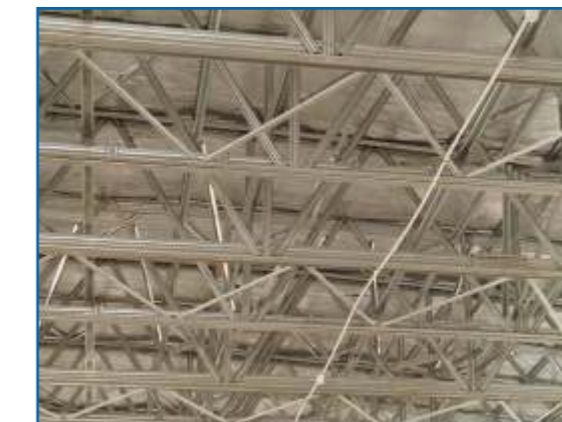
Top-Hat profiles used as bracing members in an Ultra-Span light gauge steel roof structure.
